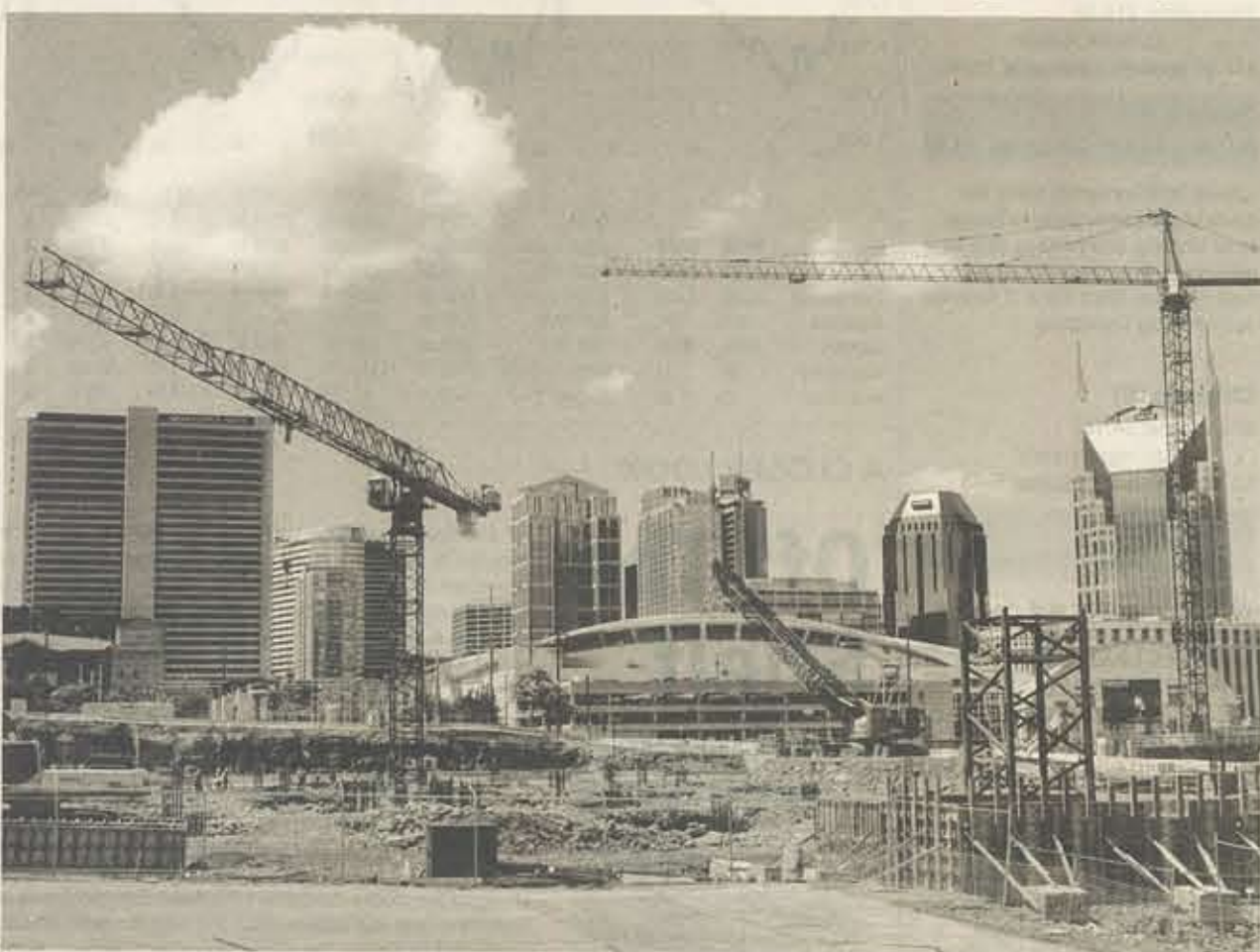
A handful of large projects around Tennessee — including work on the Music City Center in downtown Nashville — appears to be boosting construction employment this summer. SANFORD MYERS / THE TENNESSEAN
