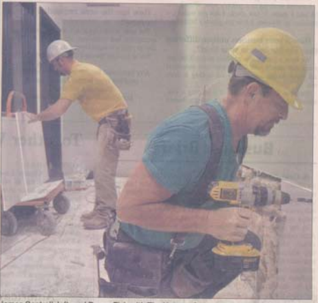
James Cantrell, left, and Danny Fish with Tim Holmes Construction are pictured putting up new drywall at F&M Bank Wednesday, a week after major flooding displaced families and flooded businesses. Another business affected in that same shopping center at the intersection of Willow and Jackson is Marble Slab Creamery. As of Tuesday, owner Rex Buckner was hoping to get that store back up and running by Friday.
