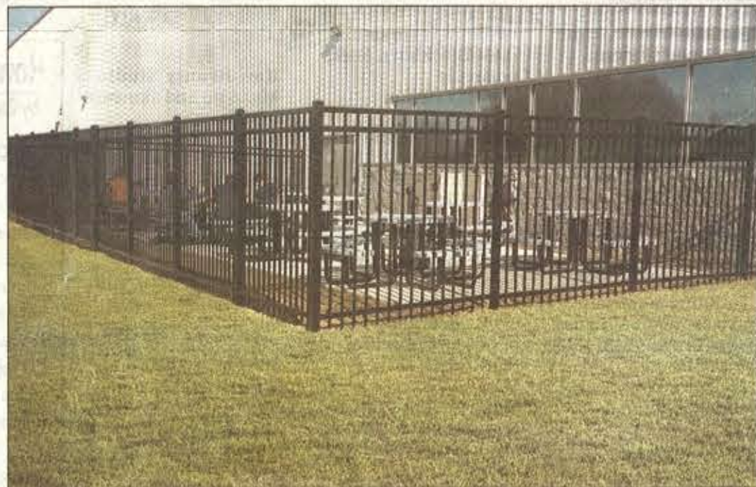
The outside fenced-in break area is one of the many projects J&S Construction recently completed at the new Ficosa plant.
